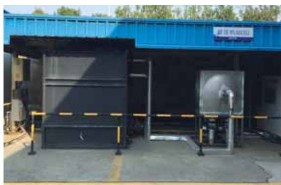
Recycling system of cooling water
