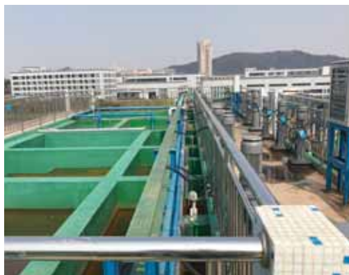
The sewage treatment plant in one of our factories in Ningbo, China
