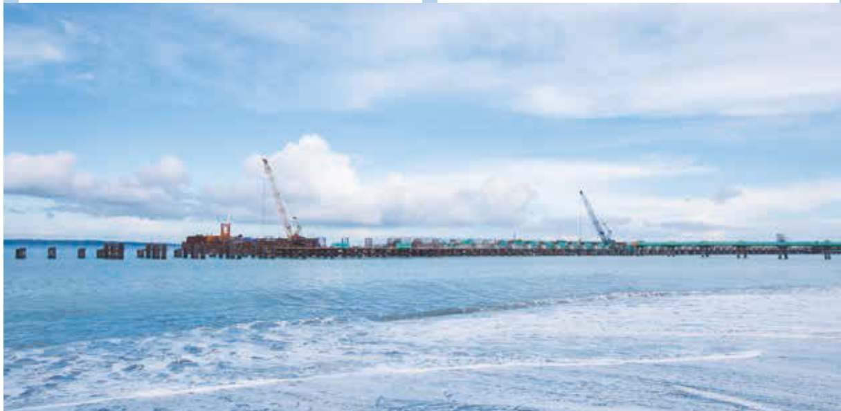
In July 2016, the terminal of the cement project in West Papua Indonesia was put into operation.
