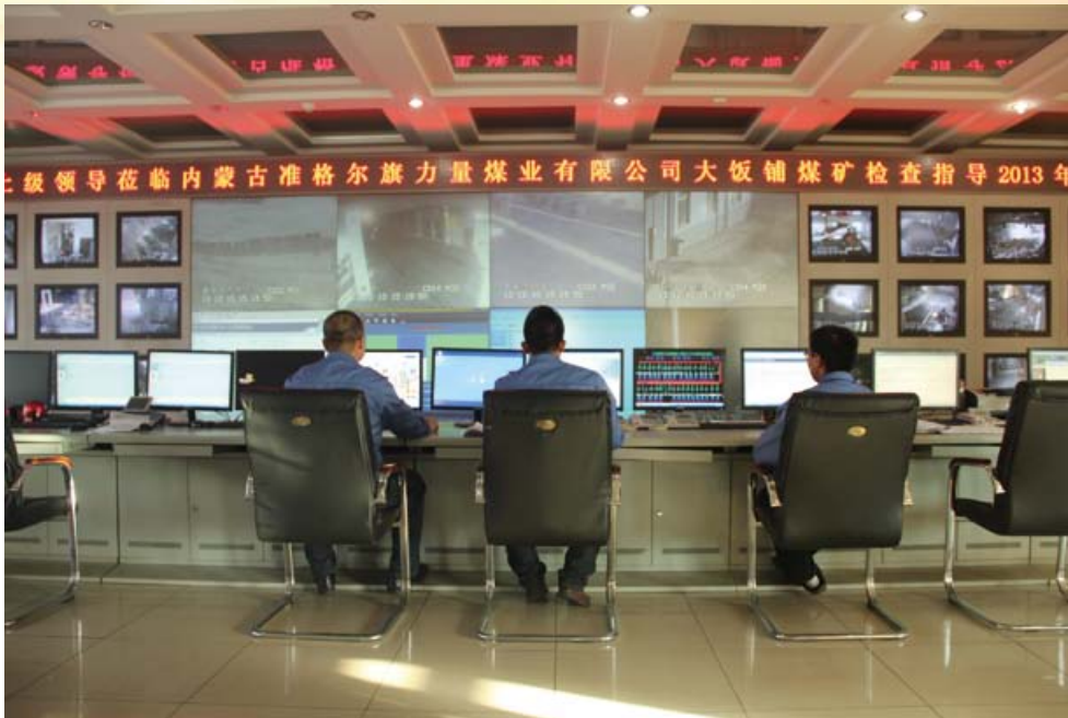
Video surveillance system in coal processing plant
