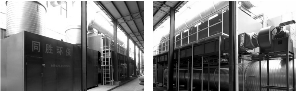
Organic air emission treatment facilities 有機廢氣處理設備
