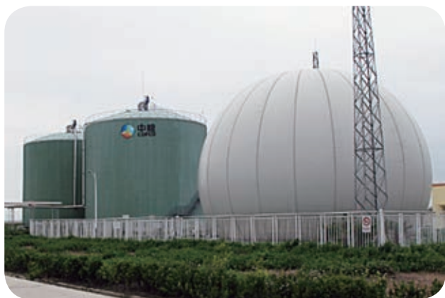
▲ Jindongtai Biogas Station of Jiangsu Company
