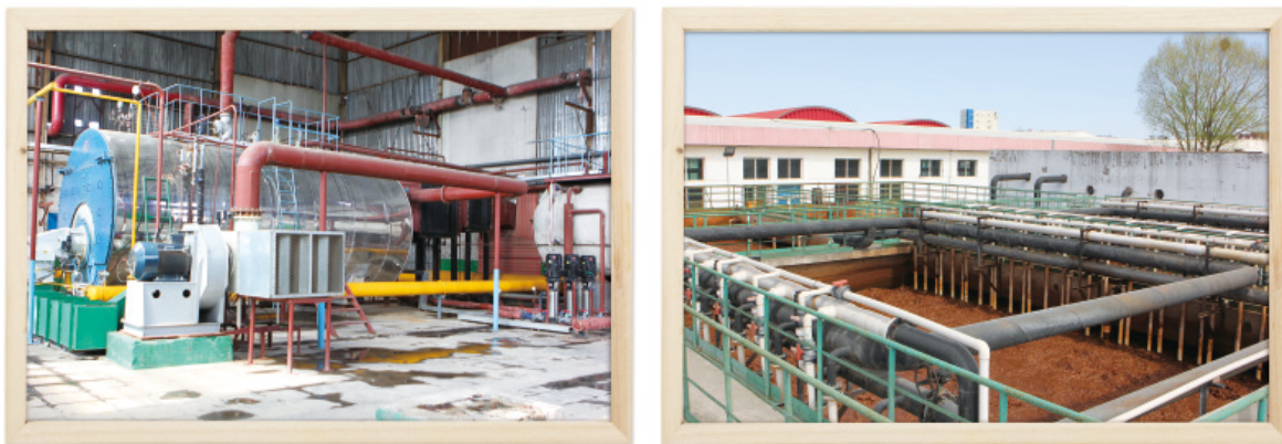
Figure 3 The gas-fired boilers and sewage treatment plant at the Group's Shunyi Plant
