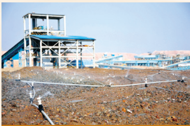
Spray leaching operations in the No.1 stockpile of heap leaching system of Muliashi Project
