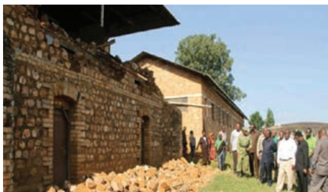
A 5.7 magnitude earthquake occurred in Kagera of North-western Tanzania, which caused many casualties, thousands of houses collapsed and road damaged
