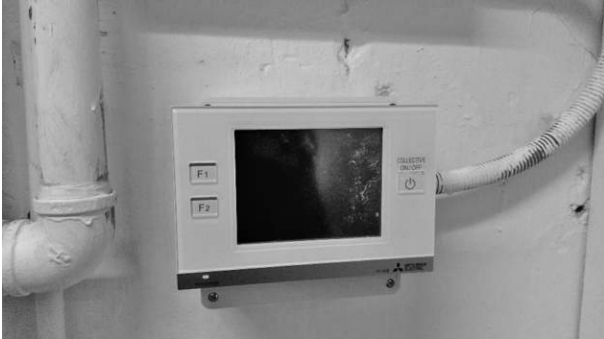
To improve energy efficiency, automated timers for both lighting and air conditioning systems have been newly installed at our Chuen Kei office in Kwai Chung.
