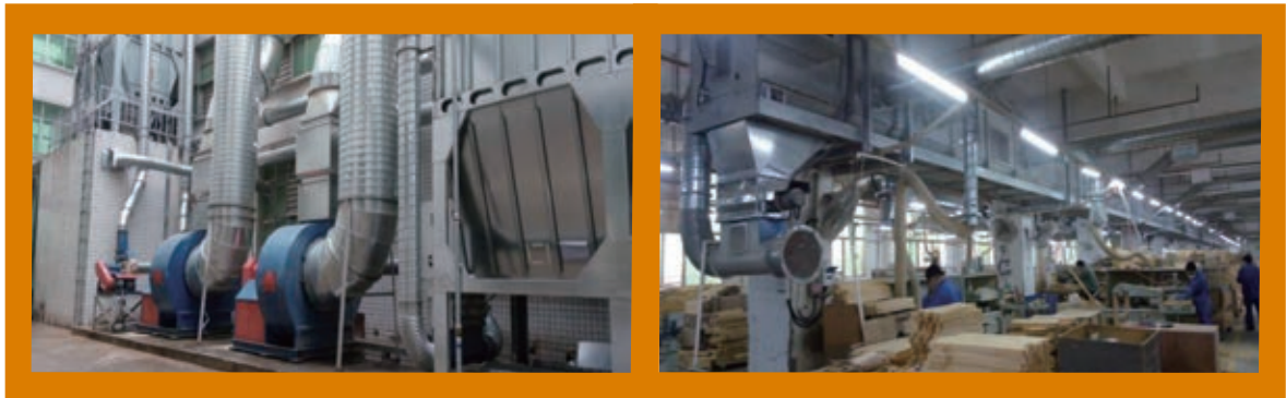
Dust Treatment Unit in Carpentry Workshop
