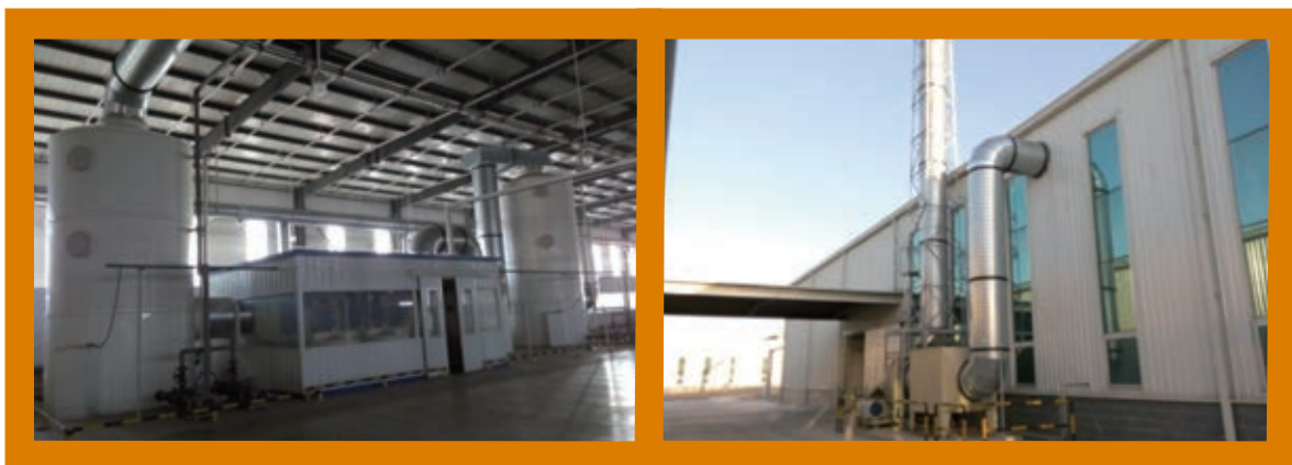
Sponge Foam Exhaust Gas Treatment Unit 1
