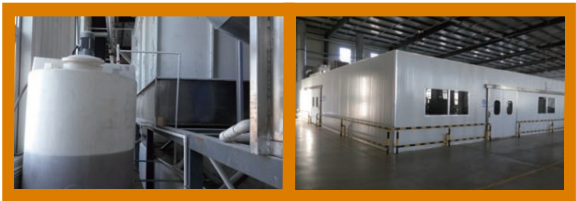
Wastewater Treatment of Panel-Type Furniture Device
