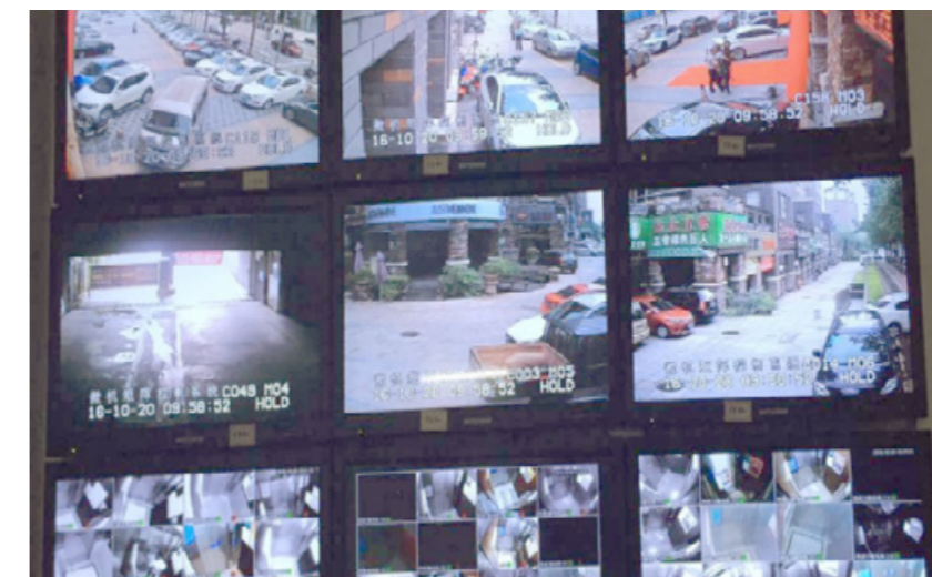
整改後的中山遠洋城監控室 Zhongshan Ocean City monitoring room after rectification
