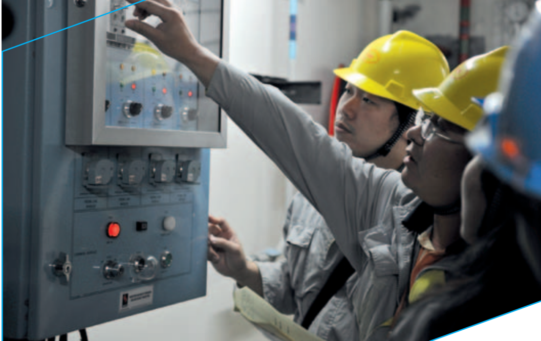
On-site inspection of equipment by operating staff
