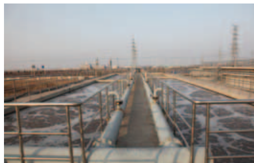
Changmao Lianyungang – Waste water processing system
