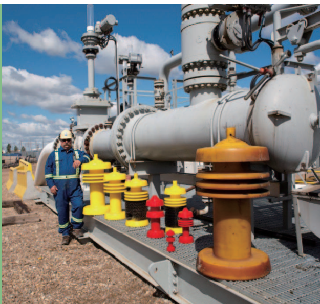
HMLP is in the process of expanding its pipeline systems to serve more customers.
