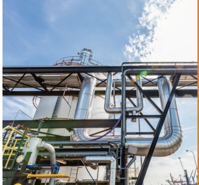
AVR's Rotterdam plant expands its supply of steam to industrial customers.
