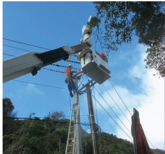
Proactive network maintenance lies at the heart of WELL's reliability record.
