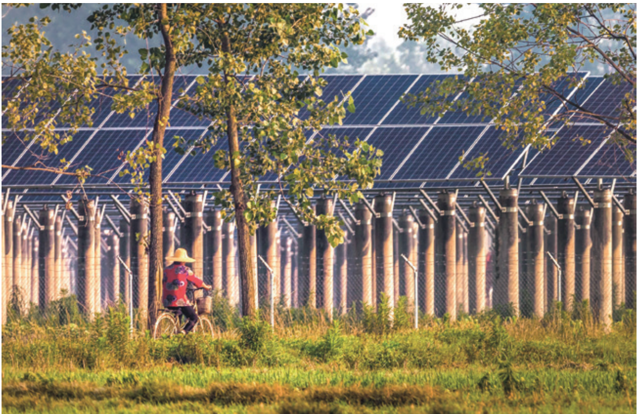
117MW Solar Poverty Alleviation Project in Funan, Anhui Province
