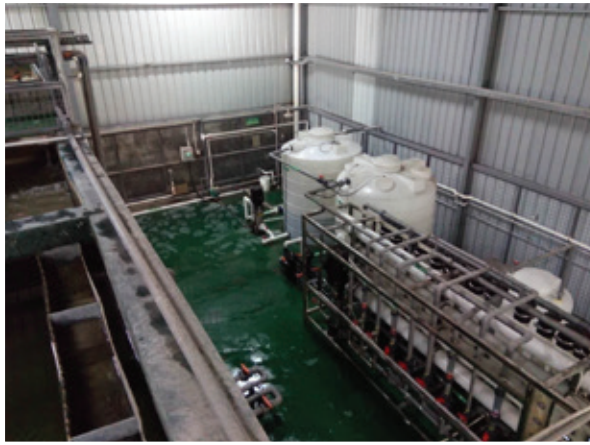
Wastewater treatment system in Ka Shui Technology's factory 嘉瑞科技廠區內之廢水處理系統
