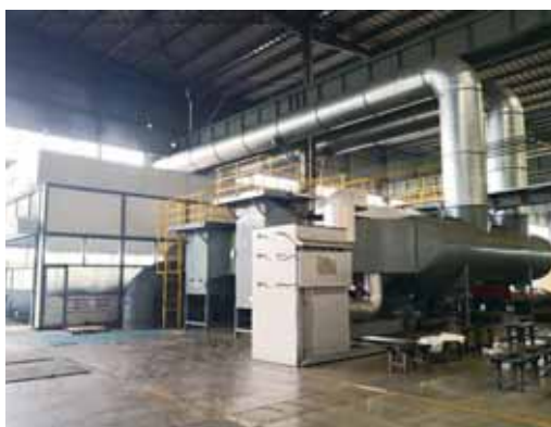
An emission processing system at a factory in Ningbo, China
