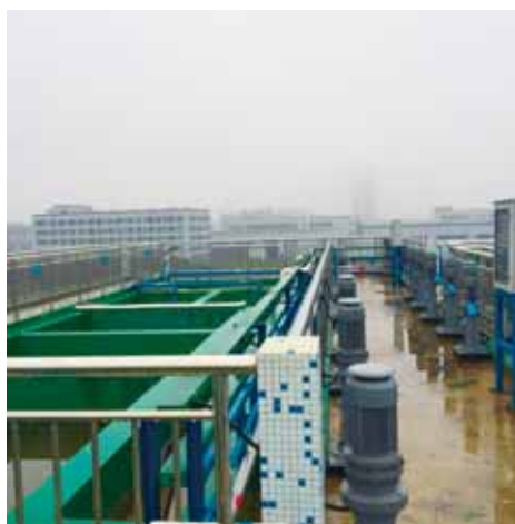
The sewage treatment plant in one of our factories in Ningbo, China
