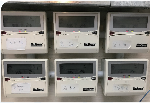
Central air conditioning system to maintain the room temperature at a steady rate 中央空調系統保持室溫穩定
