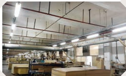
Dust Collection Unit in Carpentry Workshop 2
