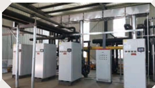
Smith EB-4000C Boiler
