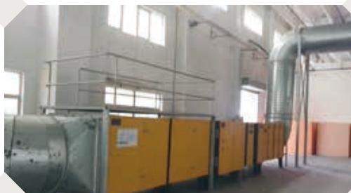
Sponge Foam Exhaust Treatment Unit 1
