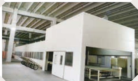
Sponge Foam Exhaust Gas Treatment Unit 2
