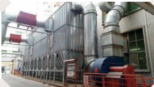
Dust Treatment Unit in Carpentry Workshop
