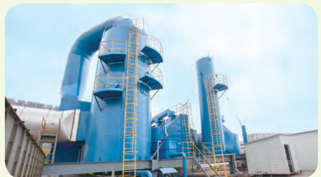
VOCs Purification System
