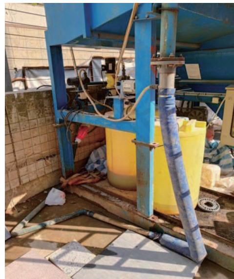
Sewage centralized for purification
