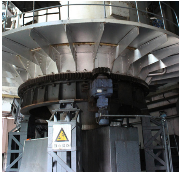
Hazardous waste incinerator 危廢焚燒爐
