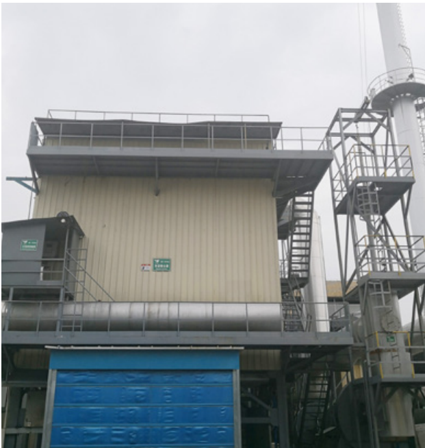
Incineration and dedusting facilities 焚燒及除塵設備
