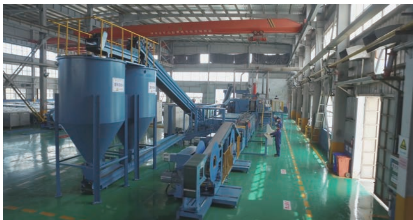
Casting and rolling production line
