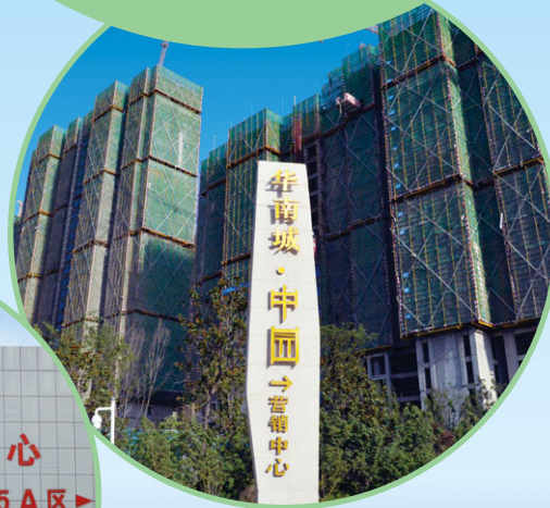
Residential ancillary under construction in CSC Zhengzhou 於鄭州華南城的在建住宅配套
