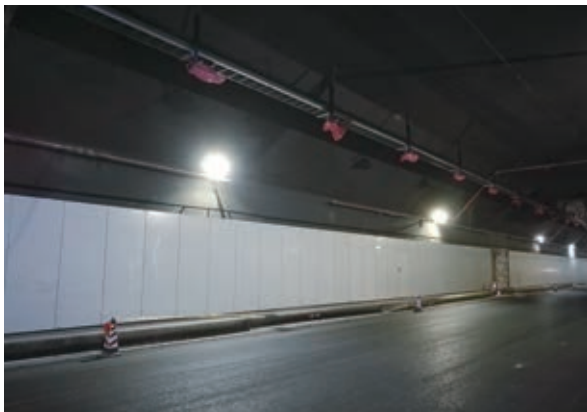
Distributed antenna systems (DAS) in subsea tunnel
