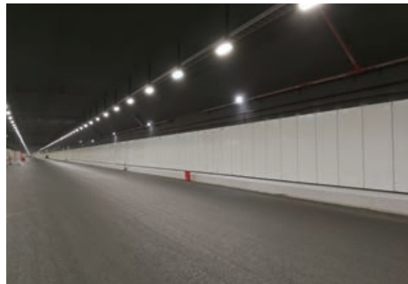
Distributed antenna systems (DAS) in subsea tunnel
