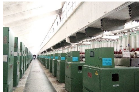
Energy Efficiency Upgrade at Changzhou Texhong 常州天虹節能改造
