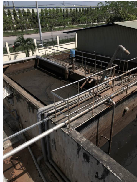
Waste water treating facilities in Dream Textile
