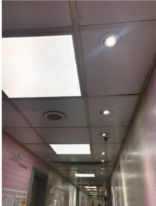
LED ceiling lights at The Langham, Hong Kong
