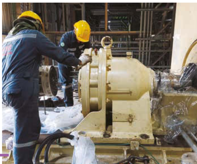
Operations in progress at RPCL.
