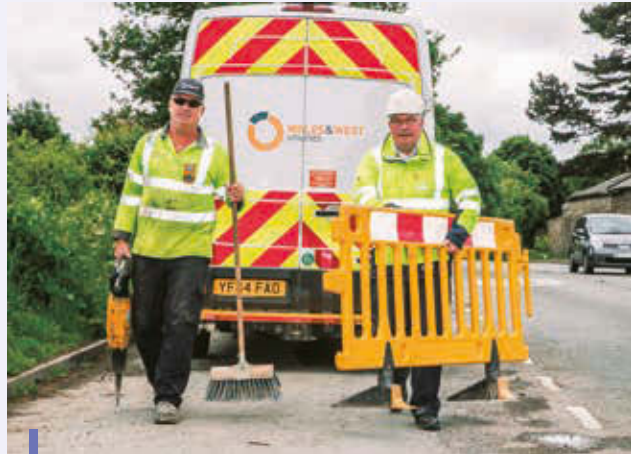
WWU colleagues at a roadside worksite. A calendar of emergency and scheduled works operates throughout the year.
