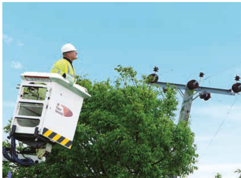
A UKPN engineer conducts maintenance on an overhead line, contributing to the company's industry-leading reliability record.
