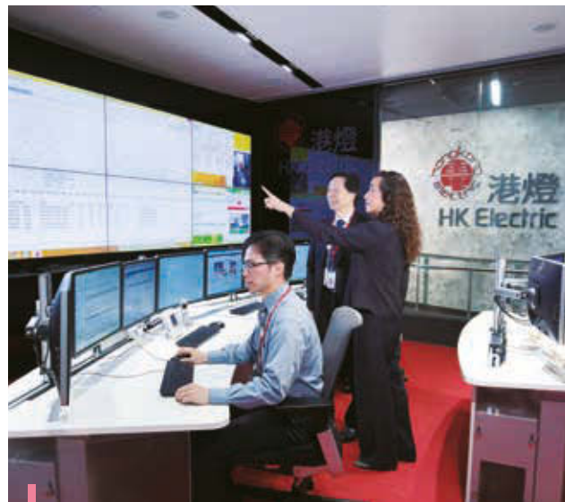
HK Electric's data centre is the nerve centre of its IT system to support non-stop operations.
