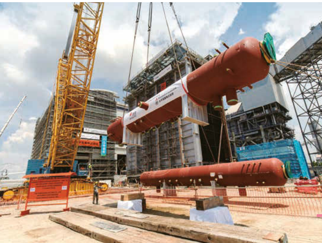
HK Electric's new L10 combined cycle gas-fired generating unit will be commissioned in 2020.
