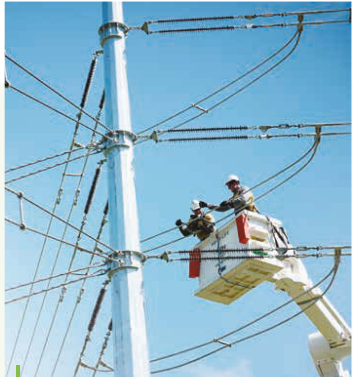
The Moorabool transmission line connecting Moorabool Wind Farm, operated by AEO.
