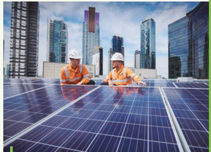
VPN's Beon Energy Solutions installing Melbourne's largest rooftop solar system at Crown Melbourne, with a capacity of 300 kW.
