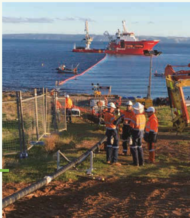
SAPN employees work on a cable from South Australia mainland to Kangaroo Island.
