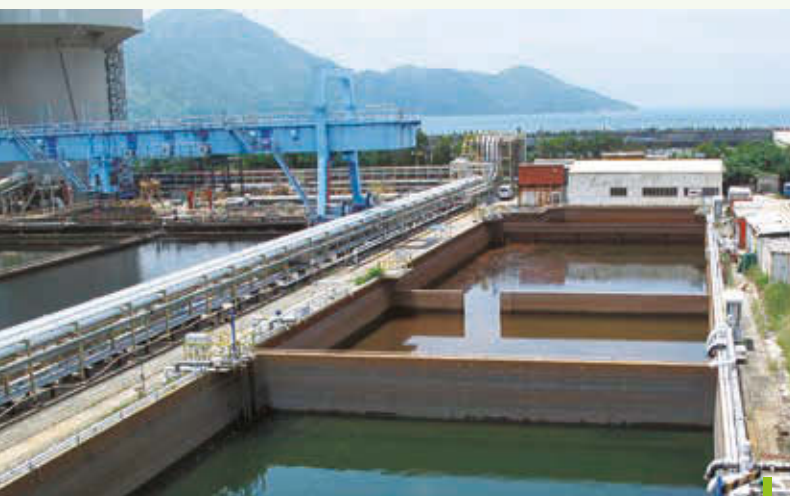
HK Electric collects and reuses recovered waste water and rain water as part of its 4R philosophy.
