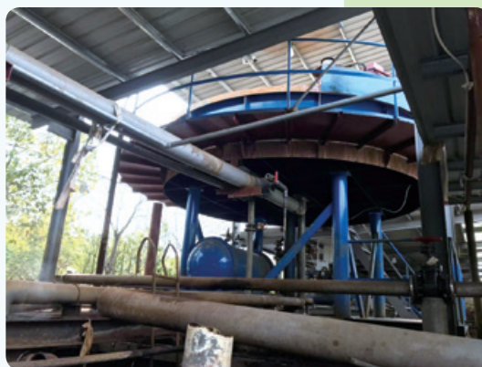
Yongsheng Dyeing's shallow air flotation system 永盛染整的淺層氣浮系統
