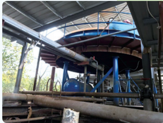
Yongsheng Dyeing's shallow air flotation system 永盛染整的淺層氣浮系統
