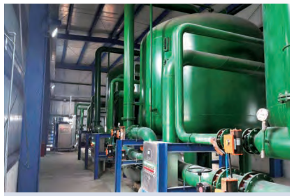
Reclaimed water treatment facilities
