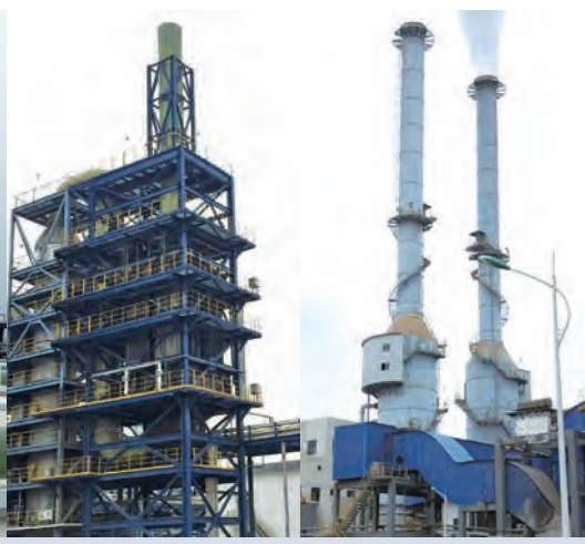
Boiler ultra low emission device
