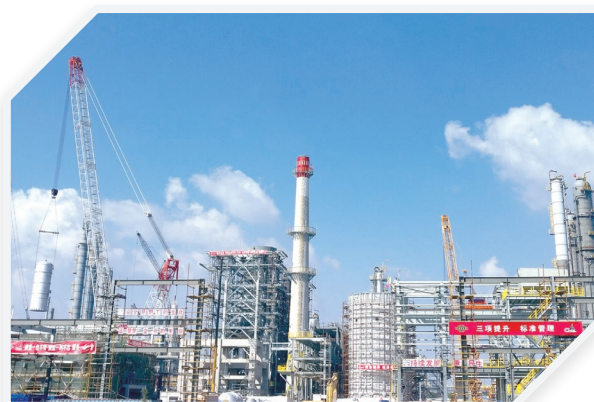
The 600kta MTO plant and the 100kta butadiene plant of Nanjing Chengzhi
