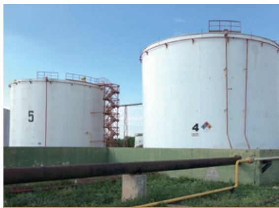
■ Oil battery tanks at Palmar Largo facility
