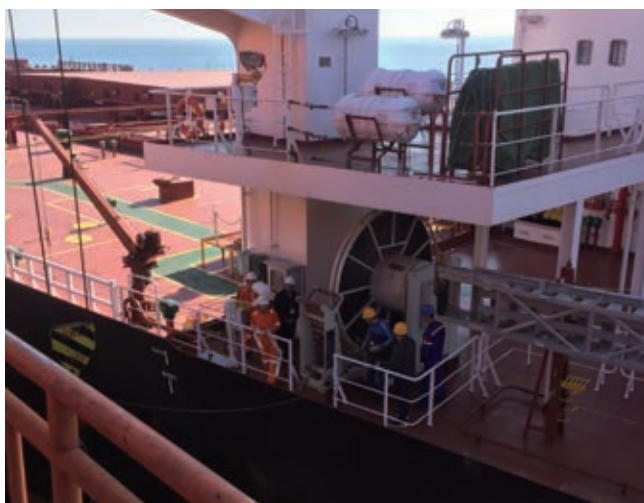
Shore-to-ship power supply equipment
