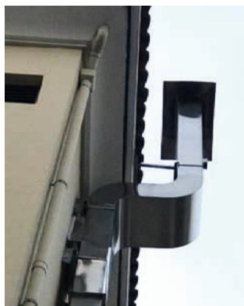
Figure: VOC ventilating chimney
