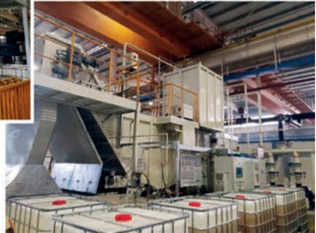
Centralized Fluid Supply system
