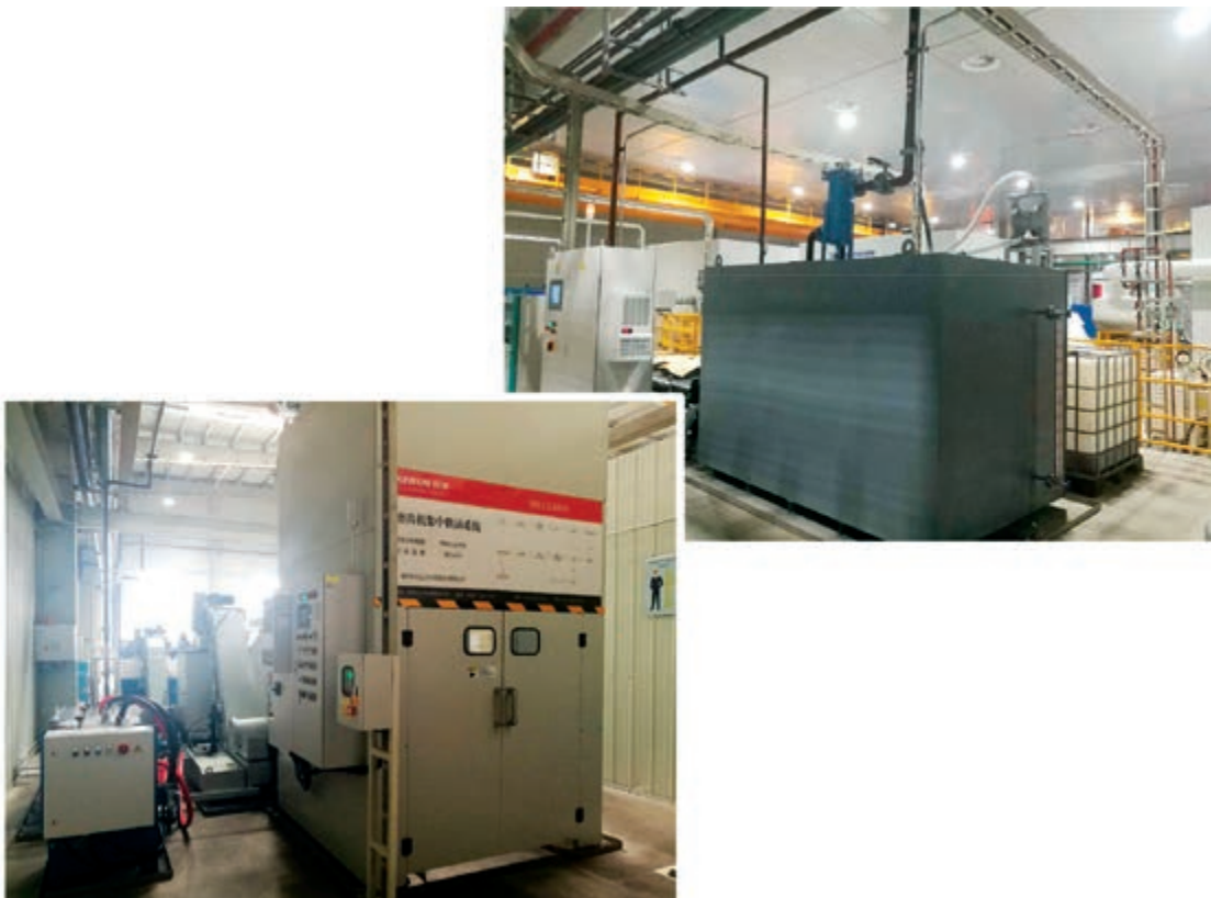
Centralized Oil Supply system
