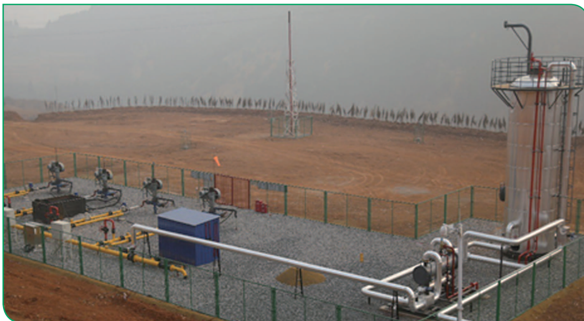
Desulfurization Tower 脫硫塔
