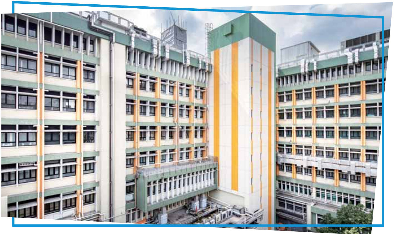
Main Contract for Refurbishment of Hong Kong Buddhist Hospital 香港佛教醫院翻新工程總合約
