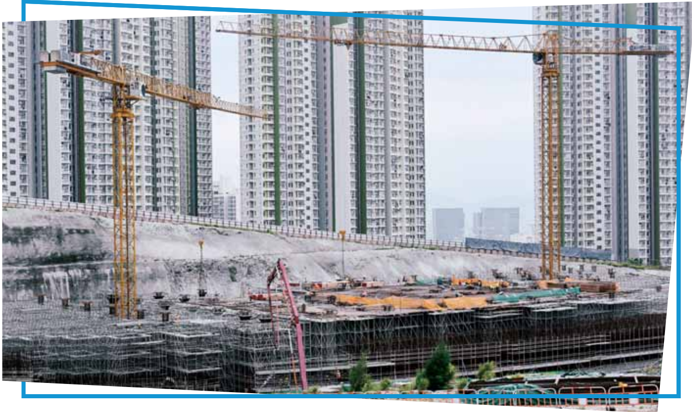
Site Formation and Infrastructure Works for Development of Anderson Road Quarry Site 安達臣道石礦場用地發展的土地平整及基礎建設工程
