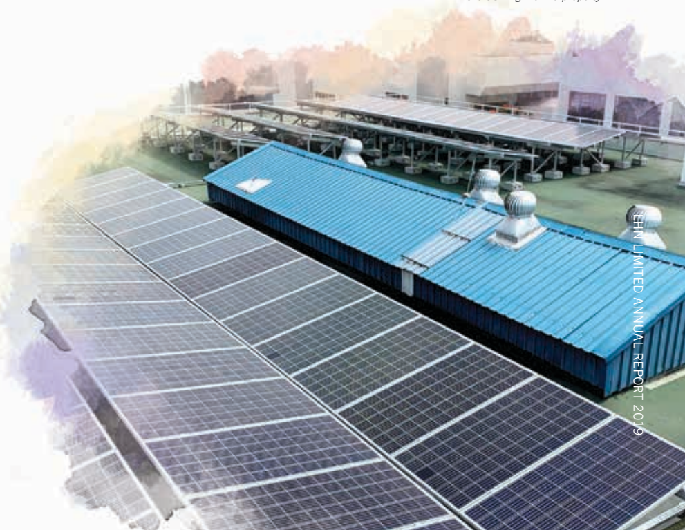
Solar panels installed at the rooftop of the 38 Ang Mo Kio property
