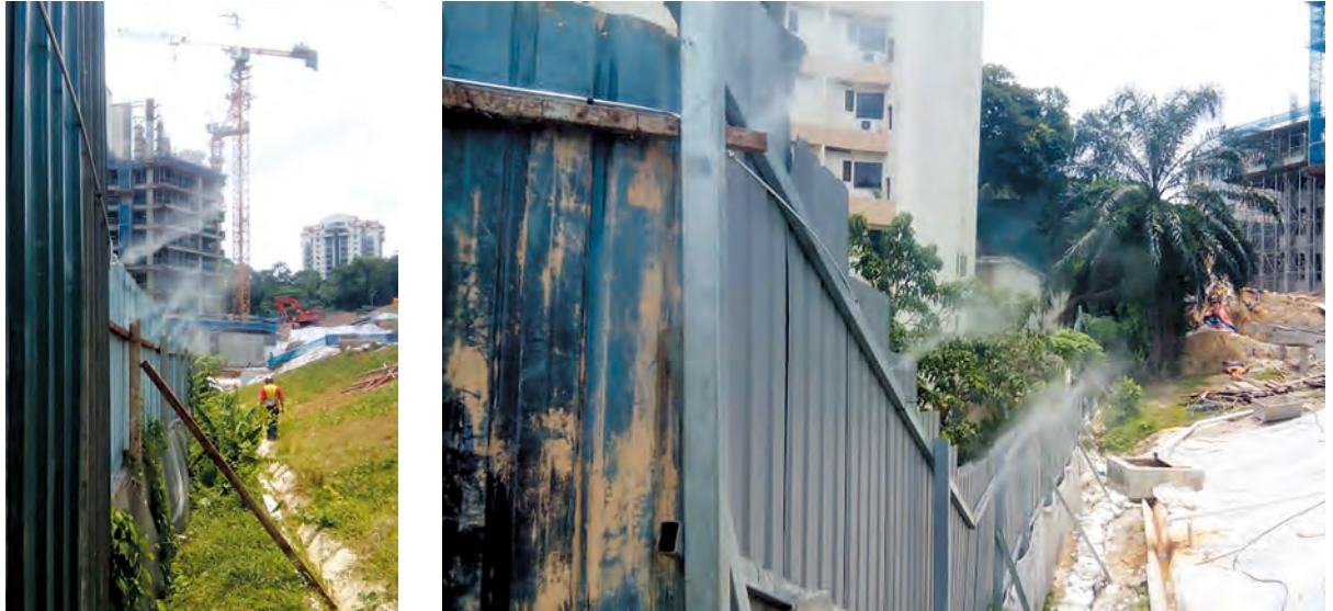
Fine mist spraying system installed along the boundary hoarding of the work site at Sky Seputeh, Kuala Lumpur. This system reduces the amount of air pollution due to dust from the construction activities to the surrounding neighbourhood.
