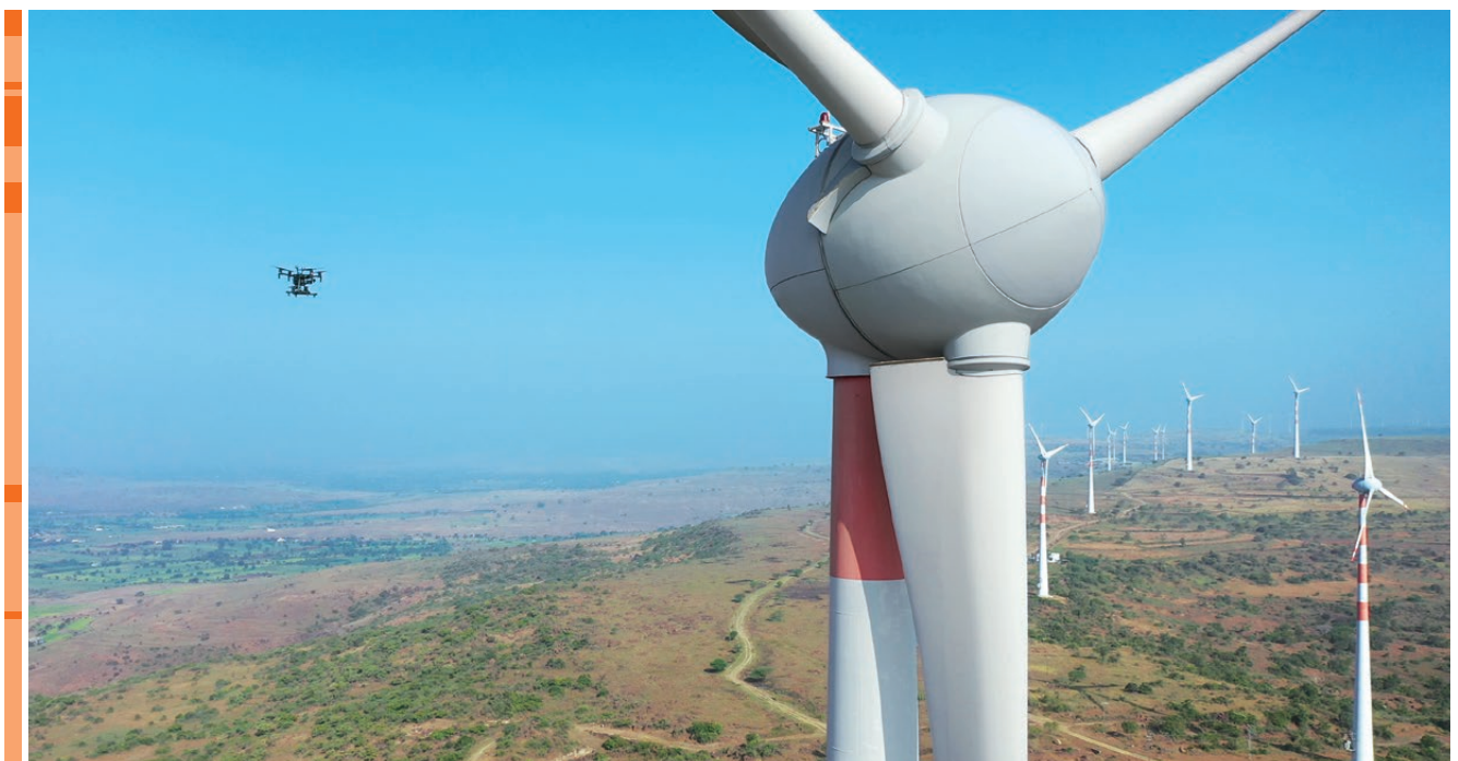
Aerial drones with high resolution cameras have been trialled for wind turbine blade inspections in India.
