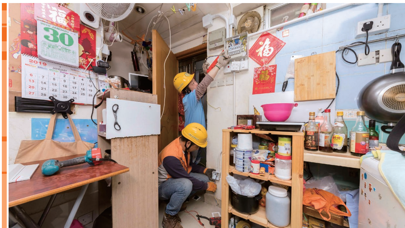
The CLP Power Connect programme in Hong Kong provides subsidies to landlords of subdivided units for rewiring work that enables installation of individual electricity meters.
