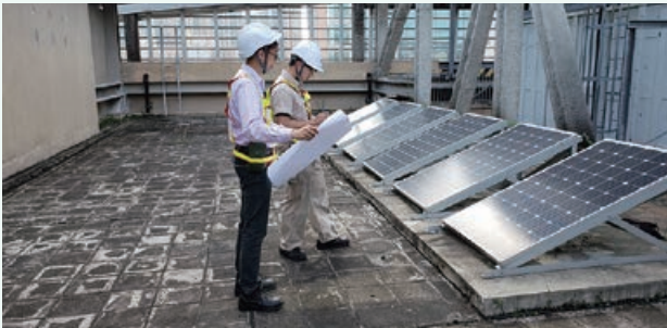
Solar panels installed on the rooftop of Langham Place Mall
