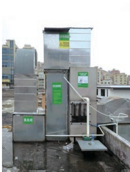
Figure: Waste Gas Treatment Facilities at Guangzhou Anmiao Shop
