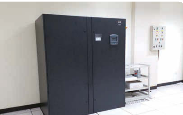
▲ Computer room air-conditioning unit at our Lamma Power Station new control building is upgraded to optimise energy use.
