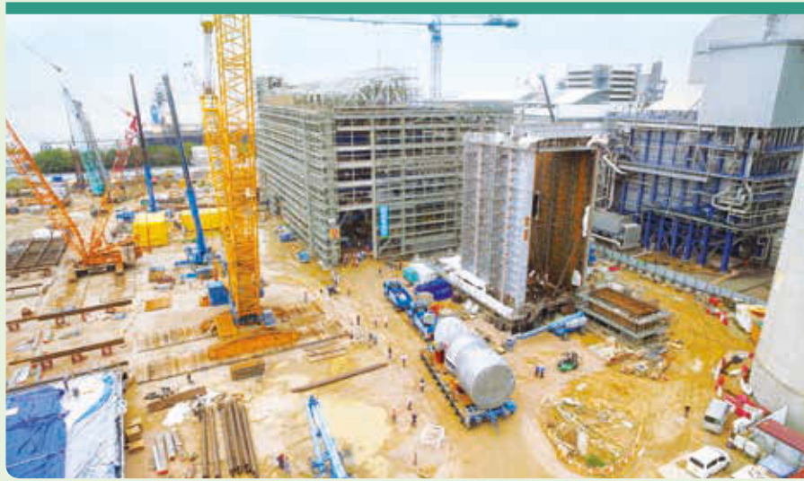
▲ Off-site fabrication allows construction to stay on track despite space constraints at Lamma Power Station.
