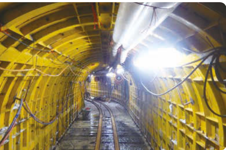
▲ The 132-kV transmission network is being extended to MTR's South Ventilation Building in Causeway Bay to support their Shatin to Central Link (Hong Kong Island Section).
