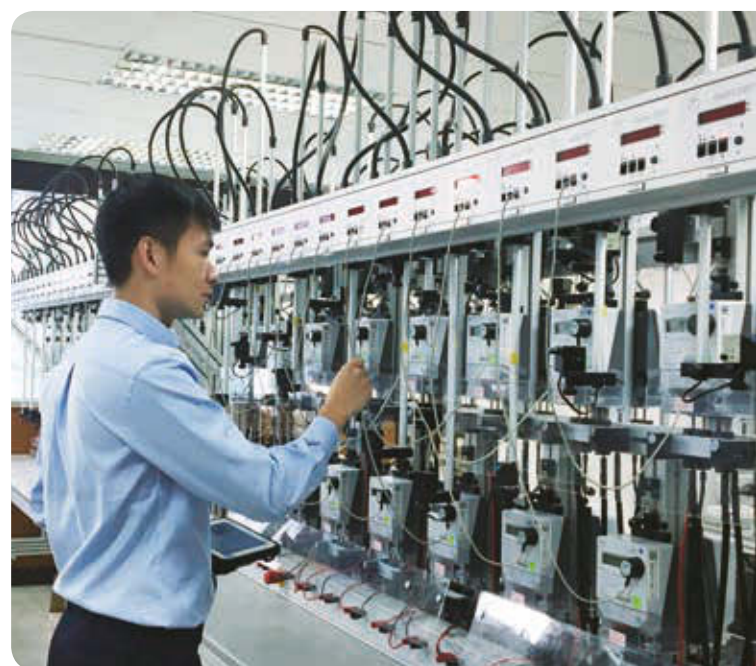
▲ Smart meters help customers improve energy management through data collection and analytics.
