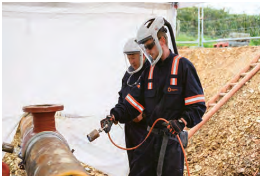
WWU engineers working on a new cross-country pipeline, which will connect a new gas-fired power site to its network.
