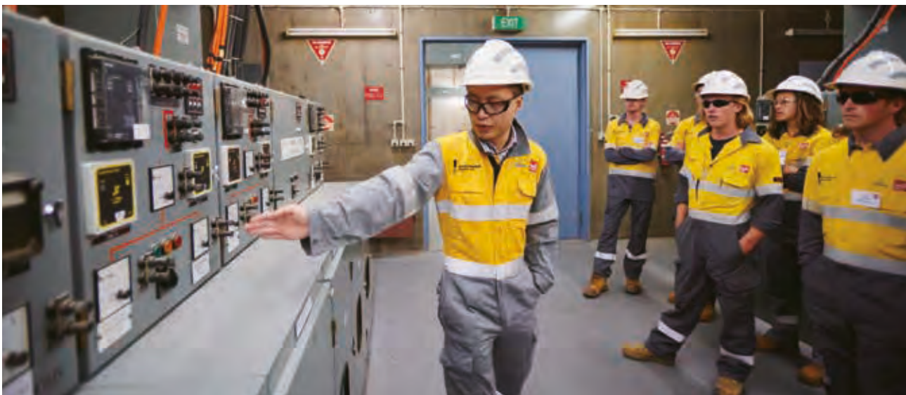
The VPN's apprentice induction and training programme includes a tour of one of the substations.
