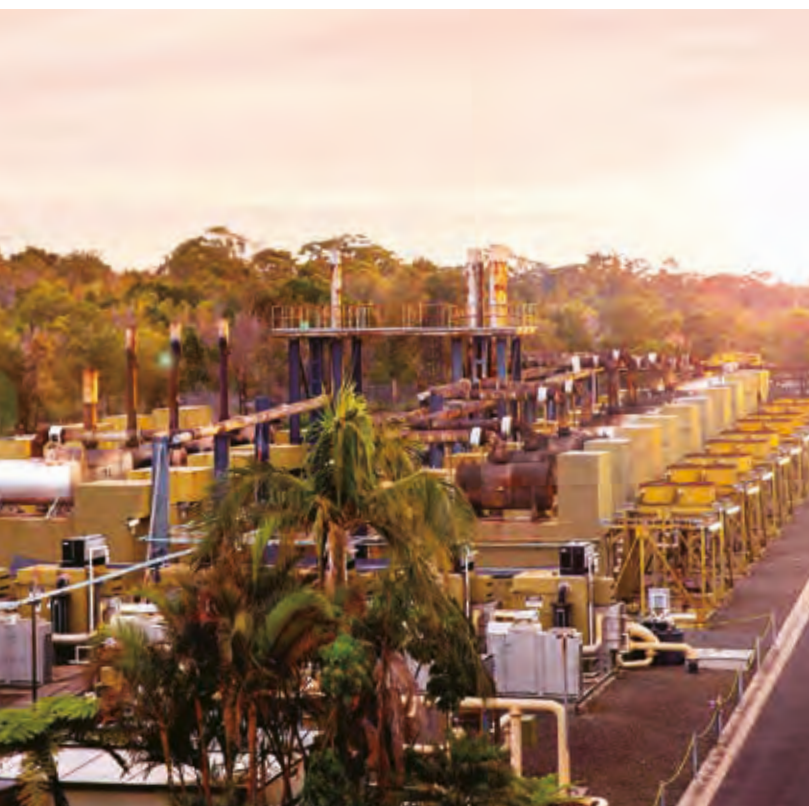
EDL's Lucas Heights power station in Australia is the venture in the Group's strategy to invest in landfill gas generation businesses.
