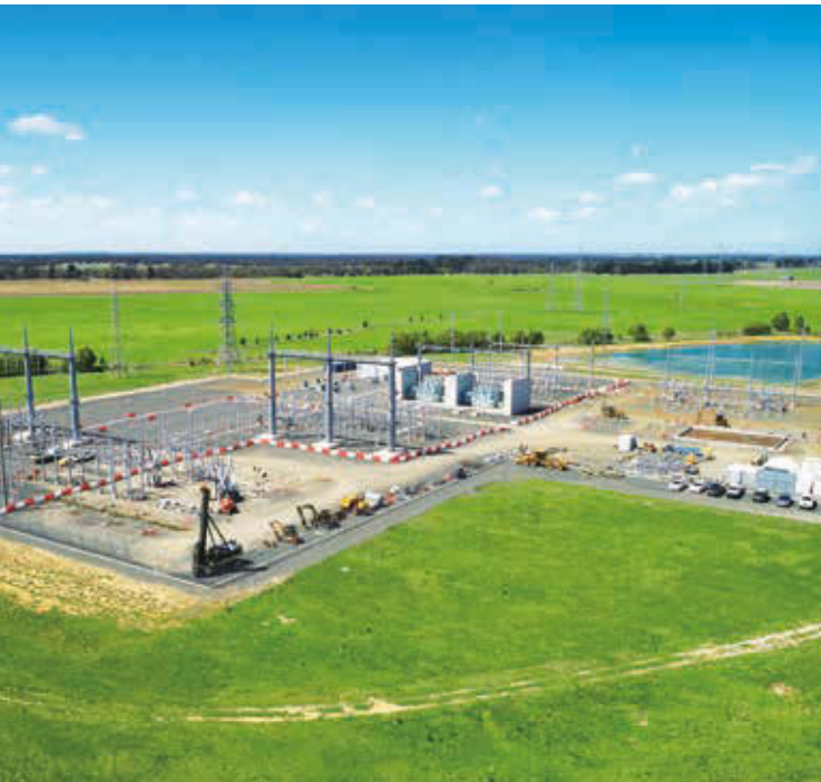
An aerial view of AEO's Elaine Terminal Station. The infrastructure connects the Elaine Wind Farm to the grid.
