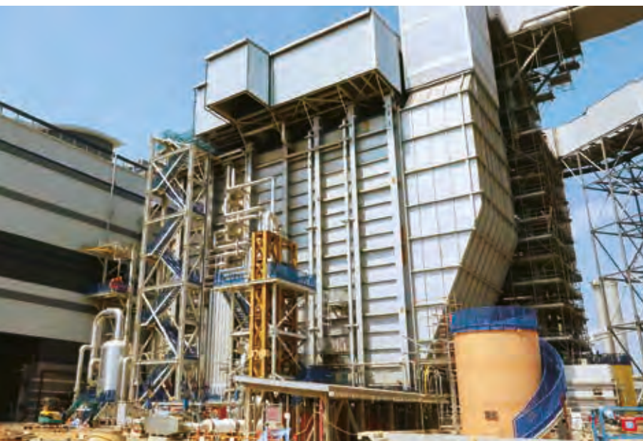
Commissioned in February 2020, HK Electric's new unit, L10, is taking the company's gas-fired generation to about 50% of total output.
