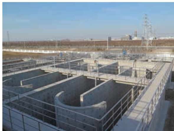
Hydrolysis Acidification Treatment System
