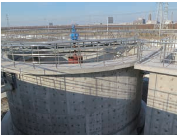
Sludge Sedimentation System
