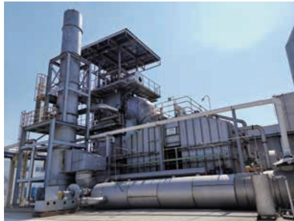
Regenerative Thermal Oxidizer (RTO) Incineration System
