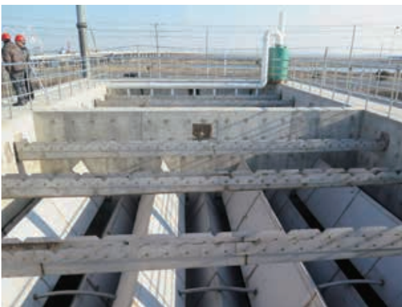
Anaerobic Fermentation Internal Components
