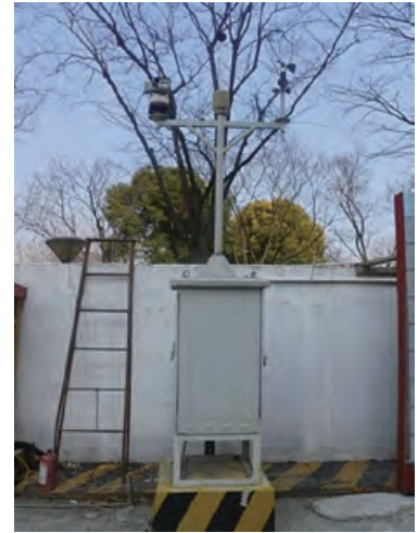
Noise dosimeters are installed at construction site to monitor noise level. Meter reading is recorded few times a day at random intervals serving as random inspections.
