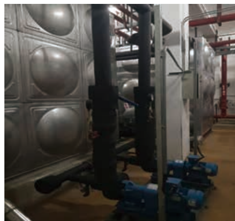
The air conditioning waste heat recovery pipelines and loop pump equipment
