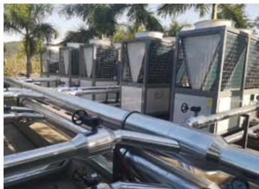
The air-energy heat pump equipment for the hot-spring thermostatic system
