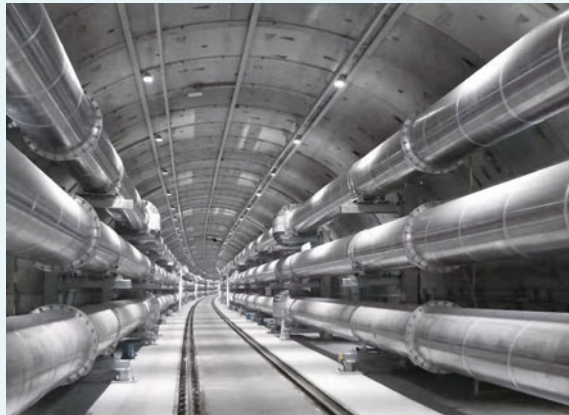
GIL outer casing of Suzhou-Nantong Pipeline
